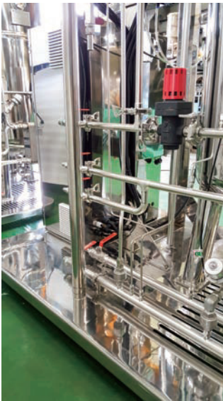
SUS316L EP Stainless Piping
